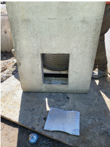
Open vault with field joint plate
